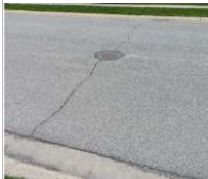
Image 1: Asphalt crack needing caulk sealing
