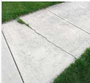
Image 2: Concrete crack & Tripping Hazard; Needing Replacement
